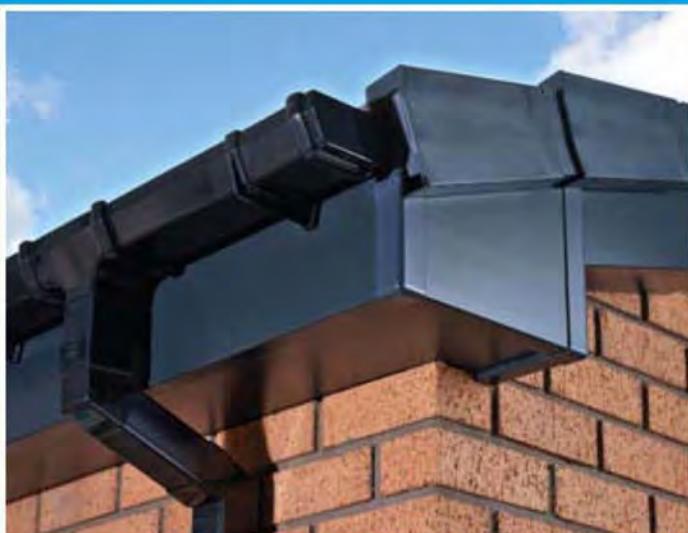
Dark Grey Fascia Black Square Rainwater
